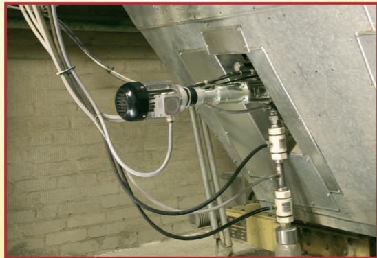
Online UBC sensor on an ash bunker.
